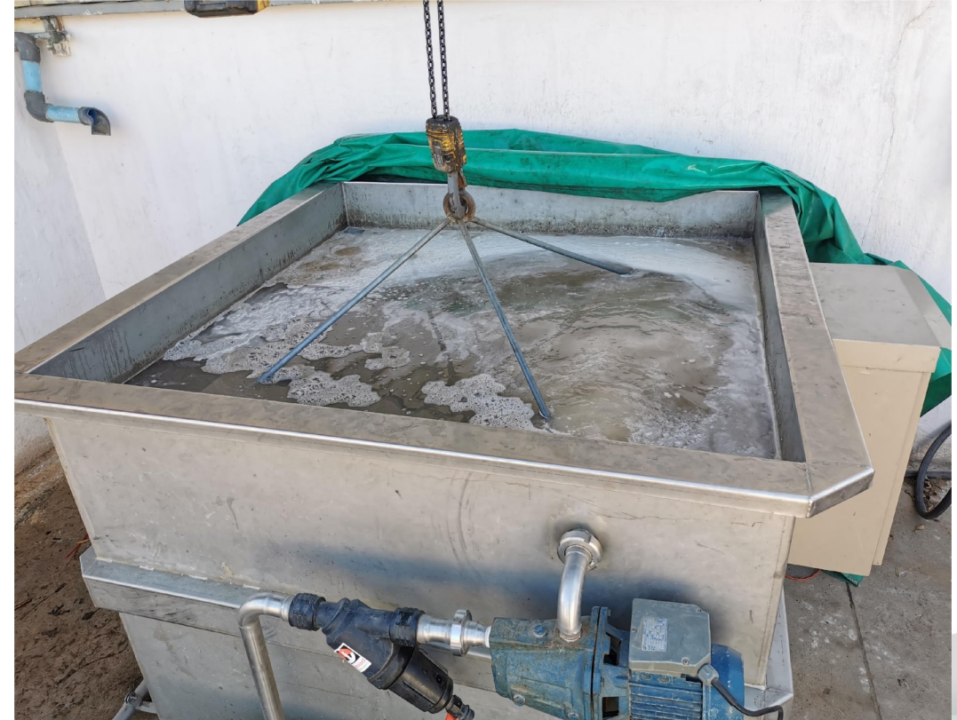
Industrial hot water treatment bath
